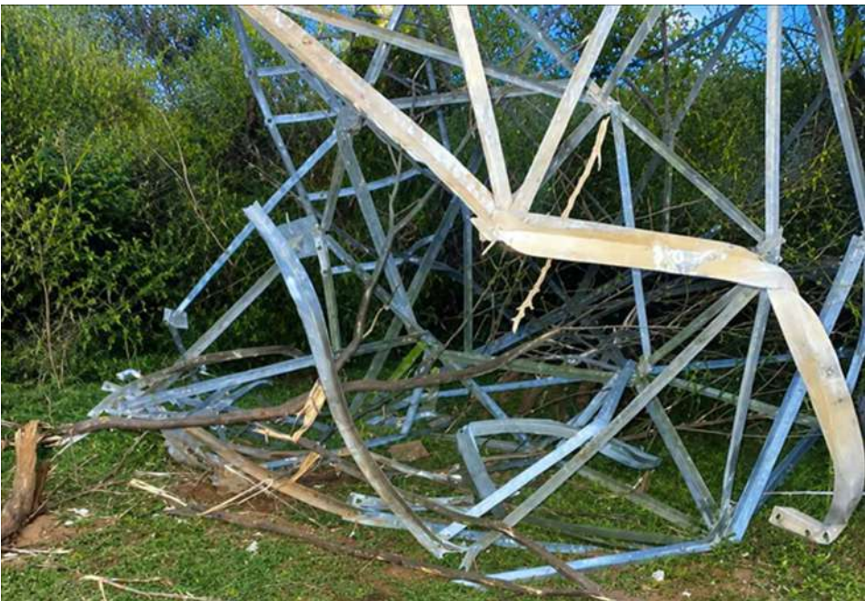
This photo shows the collapse of transmission tower No. 338 destroyed by terrorists of the 132 kV Nyaungbingyi-Buddhagon national grid on 19 July 2026.
