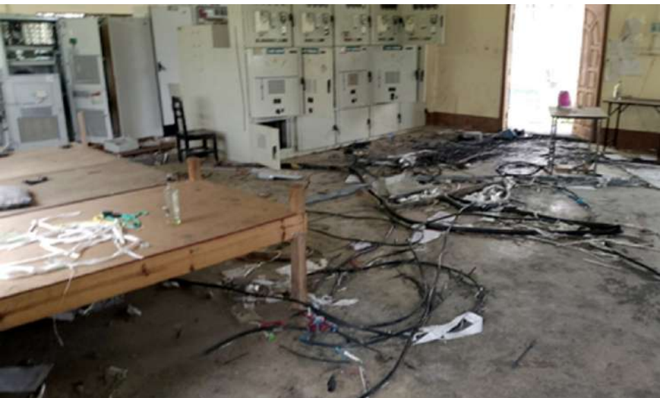
Photo records of the damage and loss at the 66/11 kV 5 MVA Falam power substation and loss of cables.
