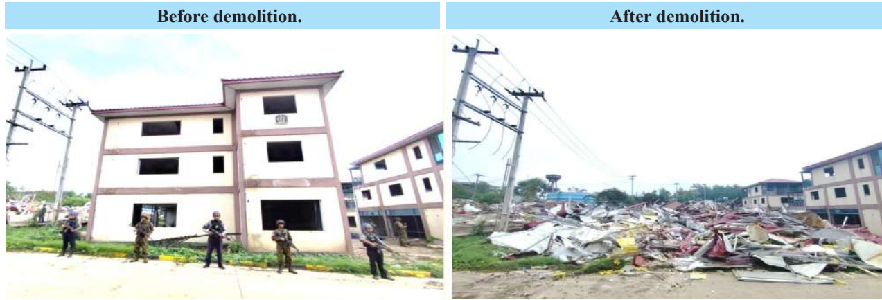
Destruction of an illegal building used for online gambling businesses in Shwe Kokko area, Myawady District, Kayin State, using machinery.
