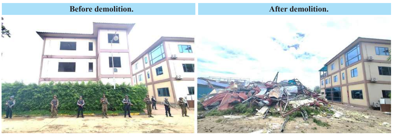
Illegal building that was used for online gambling operations in Shwe Kokko area, Myawaddy District, Kayin State, being demolished with machinery.
