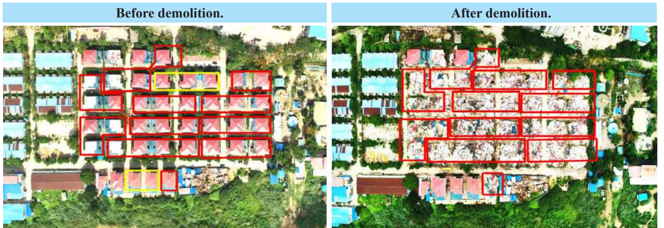
Illegal buildings that were used for online gambling operations in Shwe Kokko area, Myawaddy District, Kayin State, being demolished with machinery.
